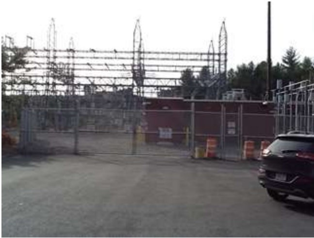
Route 11 in Franklin. Substation location houses on south side. North side has construction equipment under line then houses.
